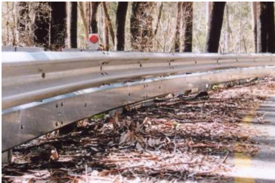
W-beam with skirt covering the posts. Lake Mountain, Victoria. October 2009.
